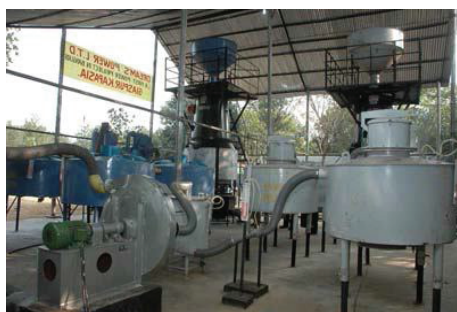
FIGURE 2: Rice husk fired 250 kW gasifier power plant at Kapasia, Bangladesh [7].
